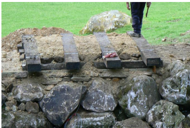
72 RECYCLED RAILWAY SLEEPERS BEING USED FOR THE CONSTRUCTION OF A BRIDGE BUTTRESS.
