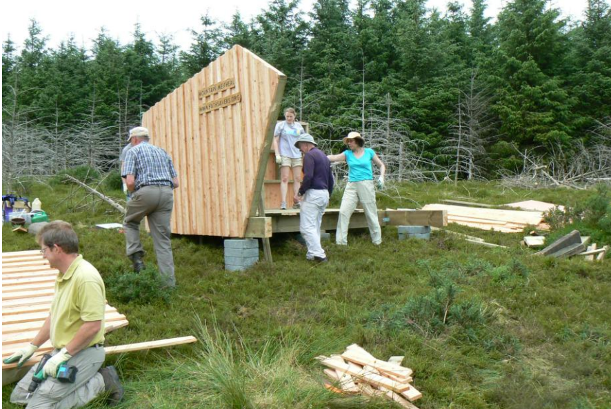
112 Keep it simple in the beginning. This trail hut constructed by Mountain Meitheal took considerable planning before the actual workday.
