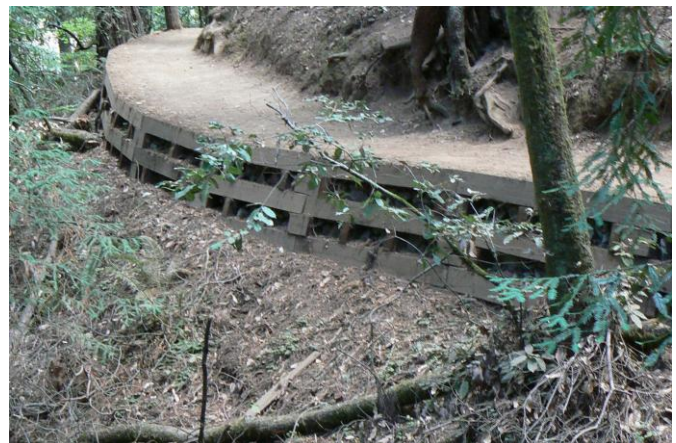
84 BUTTRESS WALL constructed from sawn timber and filled with rock rubble on a gully side slope. (Muir Woods Nat. Monument, California, USA.)
