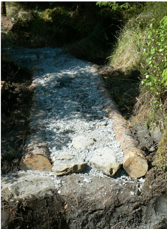
40 A COMPLETE TURNPIKE TREADWAY using log retainer walls, in-filled with large rock and finished with crushed stone.
