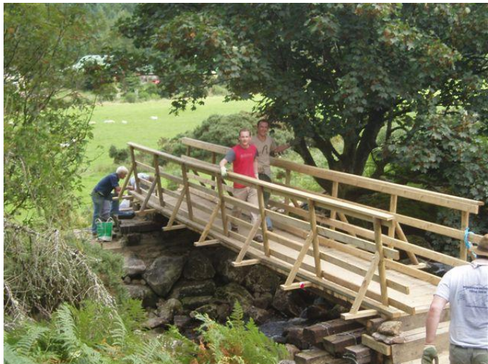
71 A FOOT BRIDGE CONSTRUCTED BY MOUNTAIN MEITHEAL IN THE WICKLOW MOUNTAINS. The bridge is built from old transmission poles and recycled railway sleepers.
