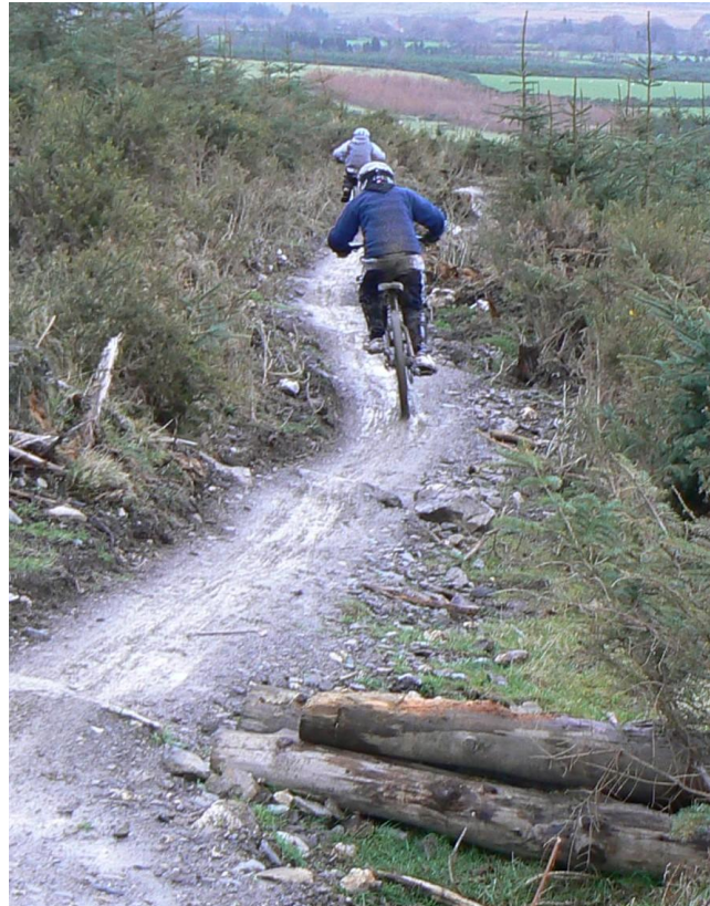
59. BENCH CUT CROSS COUNTRY TRAIL. Note the trail slopes outwards to the right to shed water off the trail. Note the use of the logs and rock to act as trail definers.
